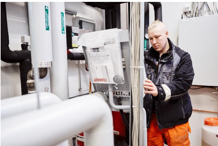
The school owns student apartments. The heat distribution room and air conditioning room in the apartments are our learning environments.
